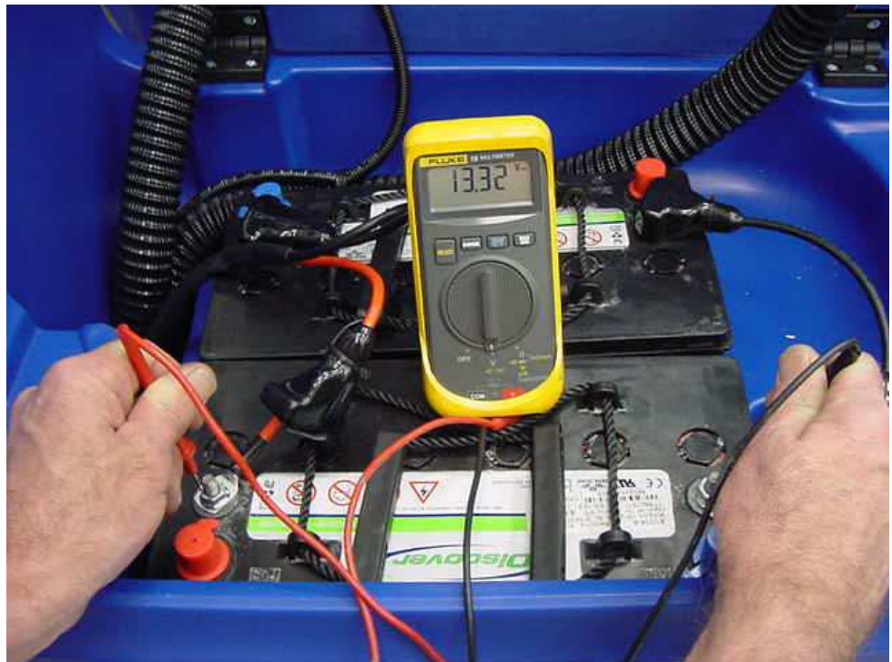
Figure 1 – Checking battery voltage (typical)
