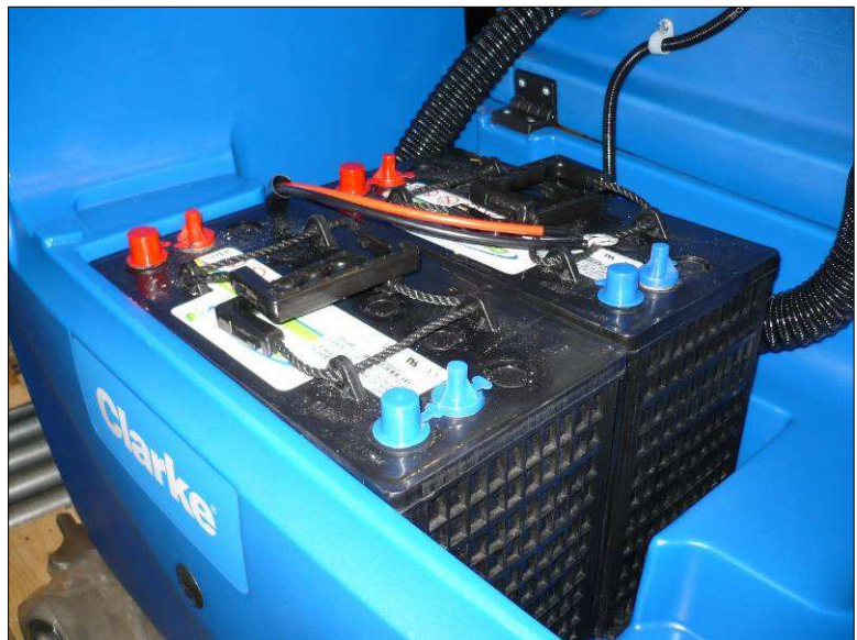
Figure 4 – Discover 140 AH EV12A Batteries
