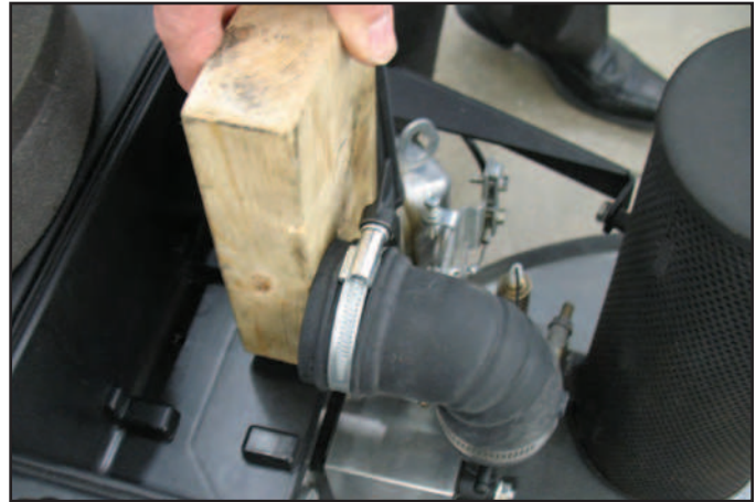
Figure 15 Partially Blocked Air Intake
