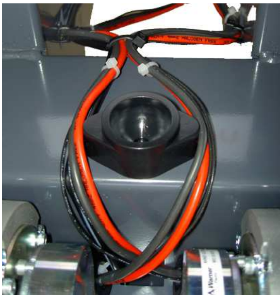
New positioning of the cables (from underneath)
